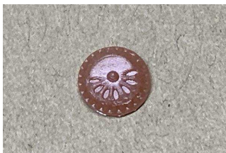
Fire Alarm Exterior
